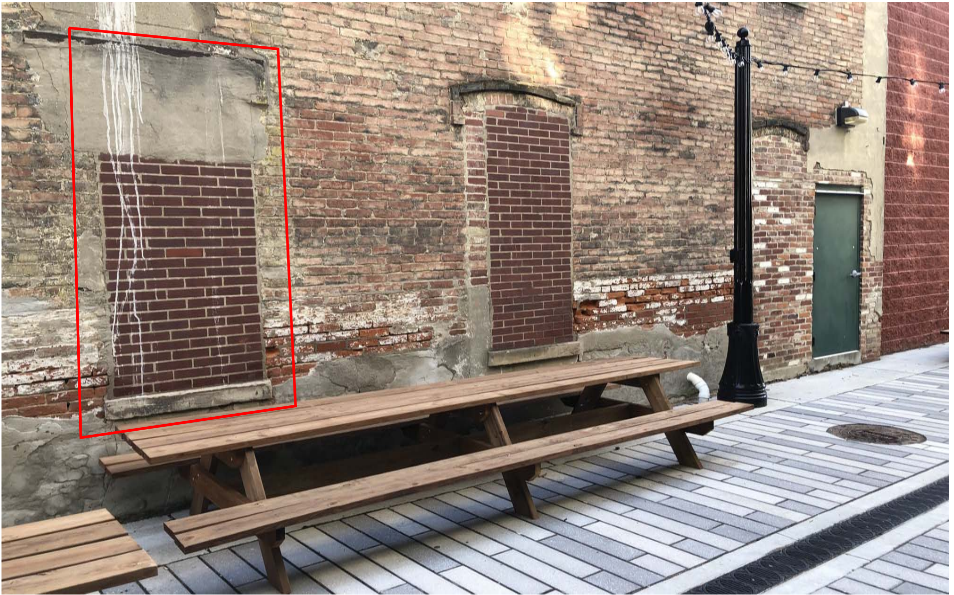
Location of replacing window. First window opening on far left. This location also lines up with the bar in the building.
